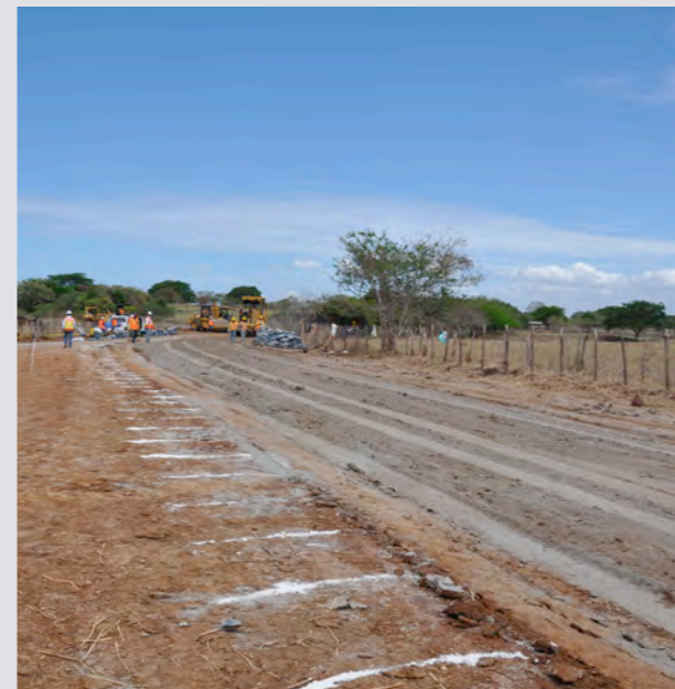
Camino El Limón road, before and after rehabilitation works (from left to right).
